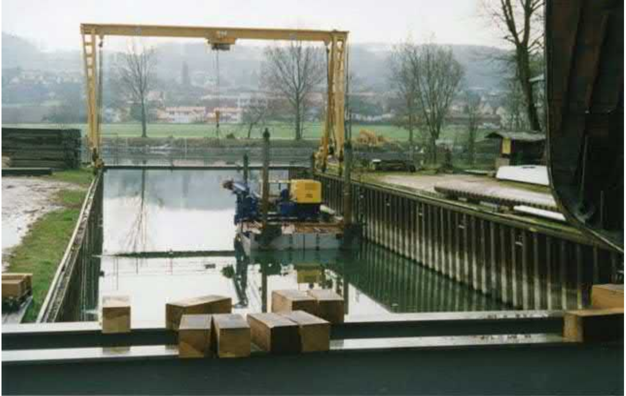
The launching place in the construction yard at Arch Photo: © Uwe Mayer / Marti AG
