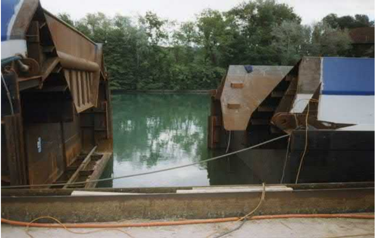
The joints of the two sections, but not jet aligned for joining
