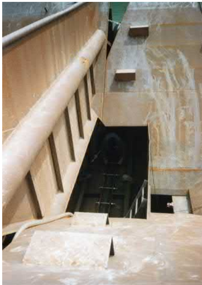
Nearing completion, one of the cargo hoppers and one of the hatches to the conveyor belt below
