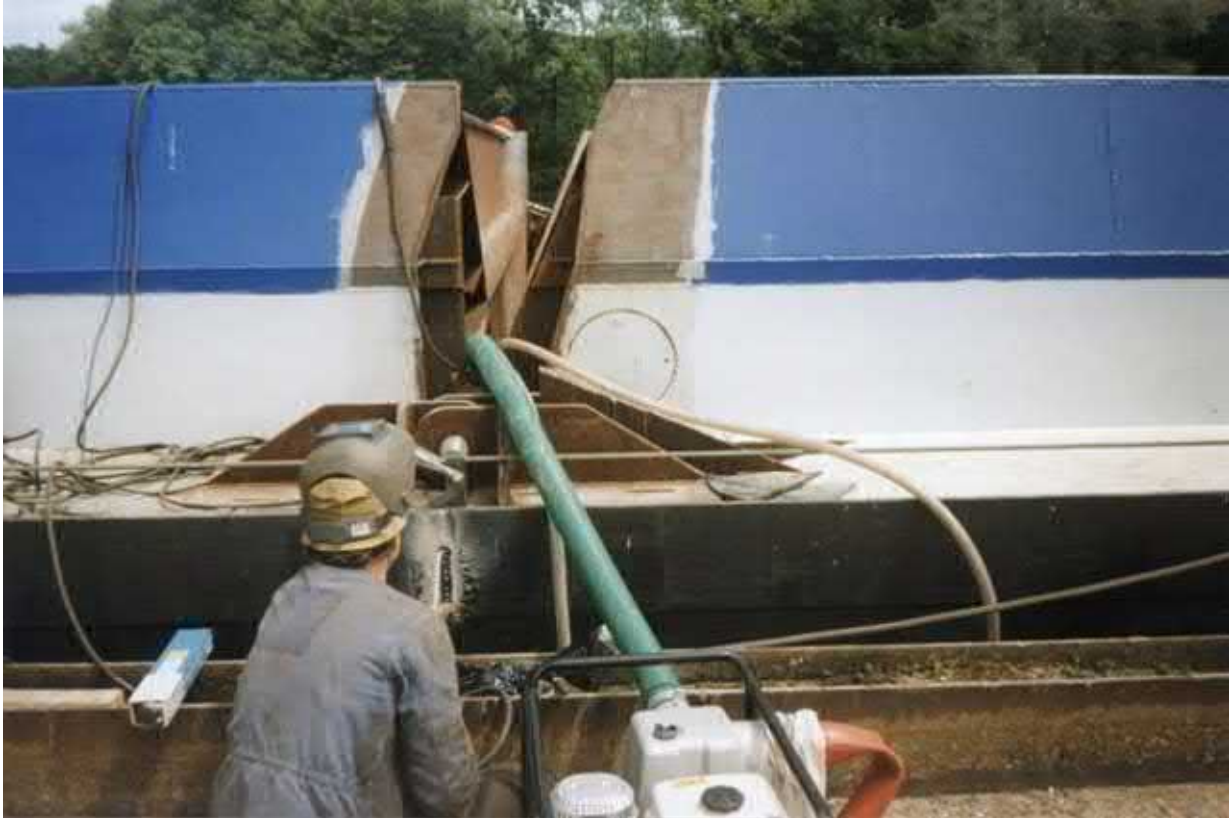
Welding in progress. Note from the interior water has to be pumped-off constantly
